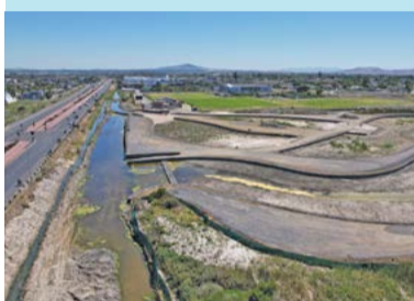
Canal's gone quiet, for now: Legal processes are under way so that work on the Bayside canal upgrade can resume with minimal delays.
