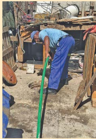
Fixers out in force: With over R1,2 billion allocated to the upkeep of the City's community residential units (CRUs) in the coming years, the municipality's 'maintenance blitz programme' attended to various essential upgrades at units in Atlantis in February.
